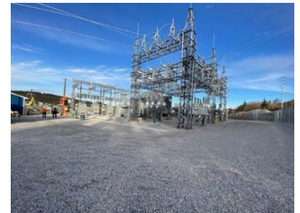
Walbournes Substation in Corner Brook.
