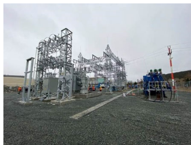
Long Pond Substation in St. John's.
