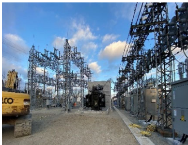
Molloy's Lane Substation in St. John's.
